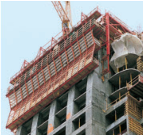
Adapting the ACS climbing units to the non-linear shape of the east side of the building involved a minimum amount of modification and without any additional crane support.
