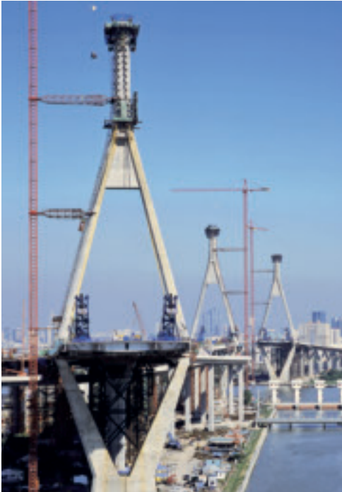
The PERI formwork solution allowed efficient construction of the complicated pylon geometry with its complex three-dimensional intersections due to forward and reverse inclinations as well as tapering cross-sections with chamfered edges.
