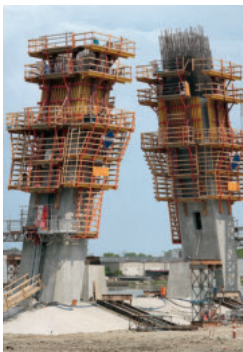
Both pylon legs were climbed simultaneously. In spite of the inclination, working platforms at all levels (concreting, main, climbing and finishing) are adjusted continuously in a horizontal position, which means construction crews can work more efficiently.
