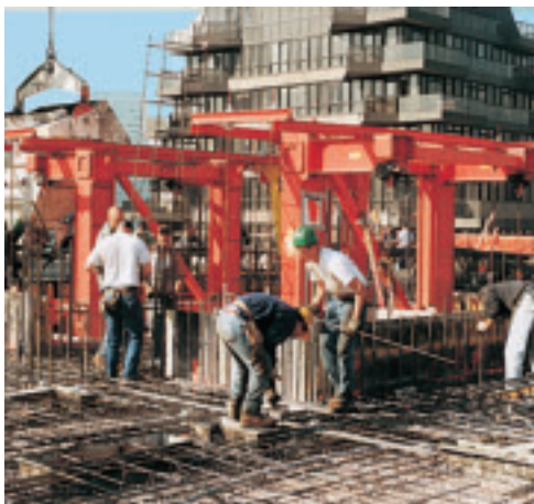
Reinforcement crew working on the upper floor layer. In the background: the gallsows of the ACS G on which the inner formwork of the core walls is suspended.
