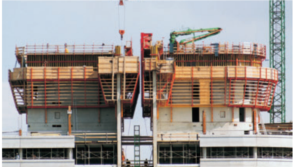
World Port Center, Rotterdam, Netherlands: A total of 25 cleverly combined ACS units (21 ACS R, 3 ACS P and 1 ACS G) provided cost-effective 5-day concreting cycles for the construction of the standard floors.
