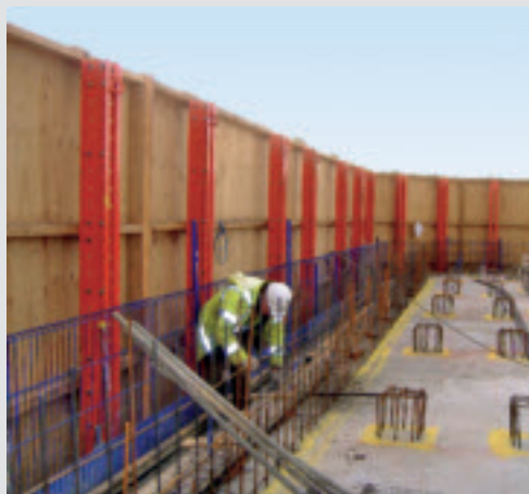
The climbing protection panel provides safe and efficient working conditions - even at great heights.
