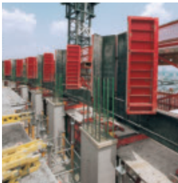
Time-saving solution: foldable steel formwork elements fixed to ACS units which climb crane-independently.
