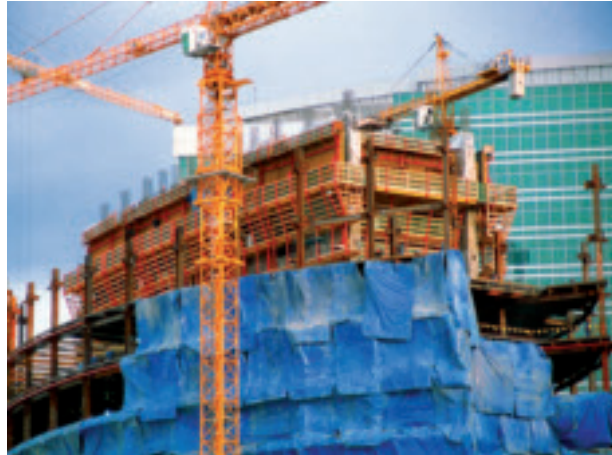
The building core with convex external walls was cost-effectively constructed in 4.30 m high concreting cycles without requiring a crane and in all weathers.
