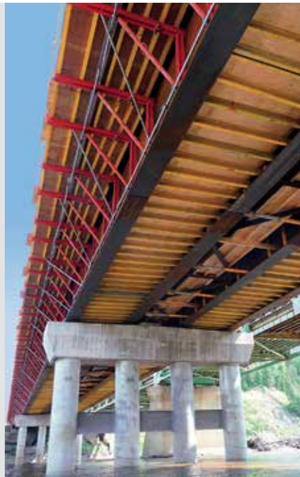
Steel composite construction method Chinchage Brücke, Canada Steel girders with in-situ concrete slabs.
