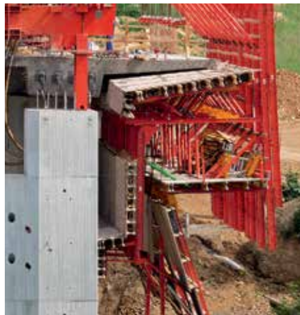
Moving past the piers is possible without any problems after the working platform and slab formwork have been hydraulically folded in.
