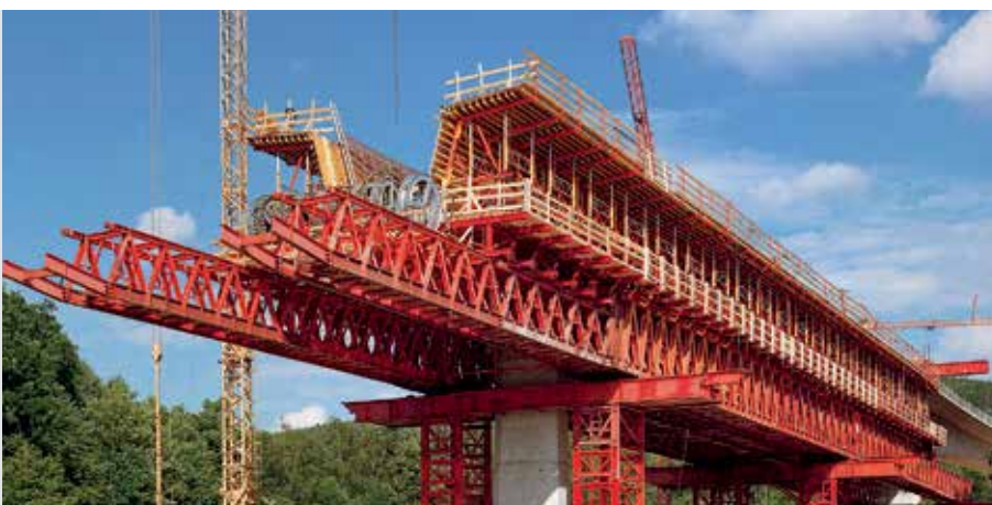
The underslung launched traveller can also be supplemented with system formwork thus ensuring cost-effective use. For moving, the traveller and formwork are firstly pushed sideways, then moved forward in a longitudinal direction and subsequently realigned.
