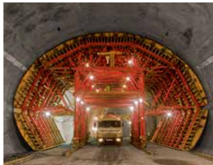
For mining tunnels, access portals are an important prerequisite for the use.
