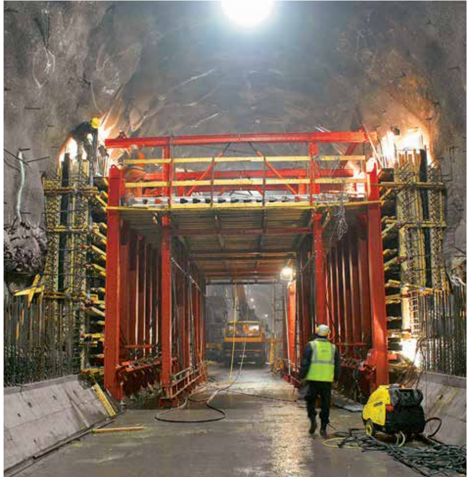
The first section with the bottom slab and starter has already been concreted.
