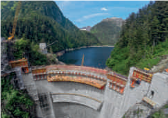
Dam upgrade project: as part of a hydroelectric power plant expansion in Alaska, the height of the dam wall was to be increased.
