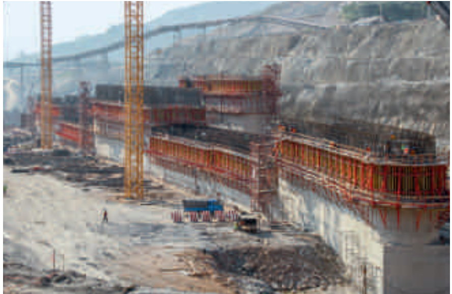
The high flexibility of the SCS Climbing System allowed an easy adaptation to suit all geometries in this dam project.
