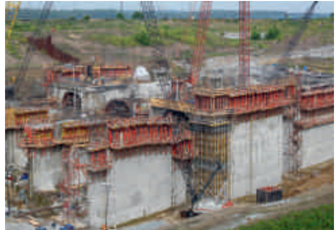
The massive power plant walls were single-sidedly formed and concreted using the SCS Climbing System.
